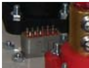
Generator alarm and control connection
